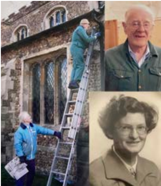
Pam and Don painting church downpipes with anti-theft paint after loss of lead from the roof.
